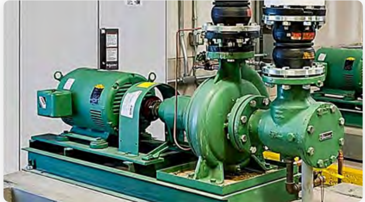
Misalignment is critical in direct coupled machines (with coupling)
