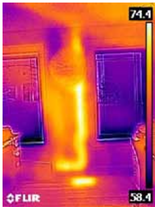
Warm drain pipe in wall
